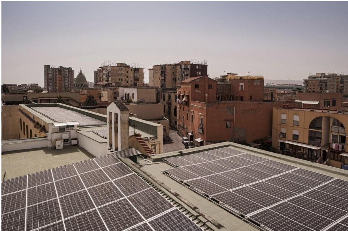
Photo 3 Maria Family Foundation roof, East Naples Energy and Solidarity Community solar panels (Legambiente photo archive)
